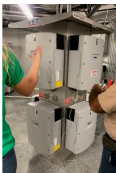
"Sunny Boy" inverter turns DC current from roof panels into AC
