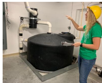
Indoor cistern; three others are outdoors underground
